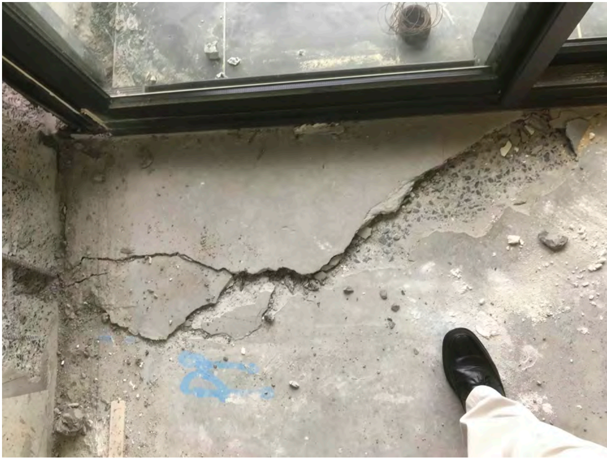
Figure 9. Photographs of the damaged floor slab adjacent to column C21 on Level 10.
