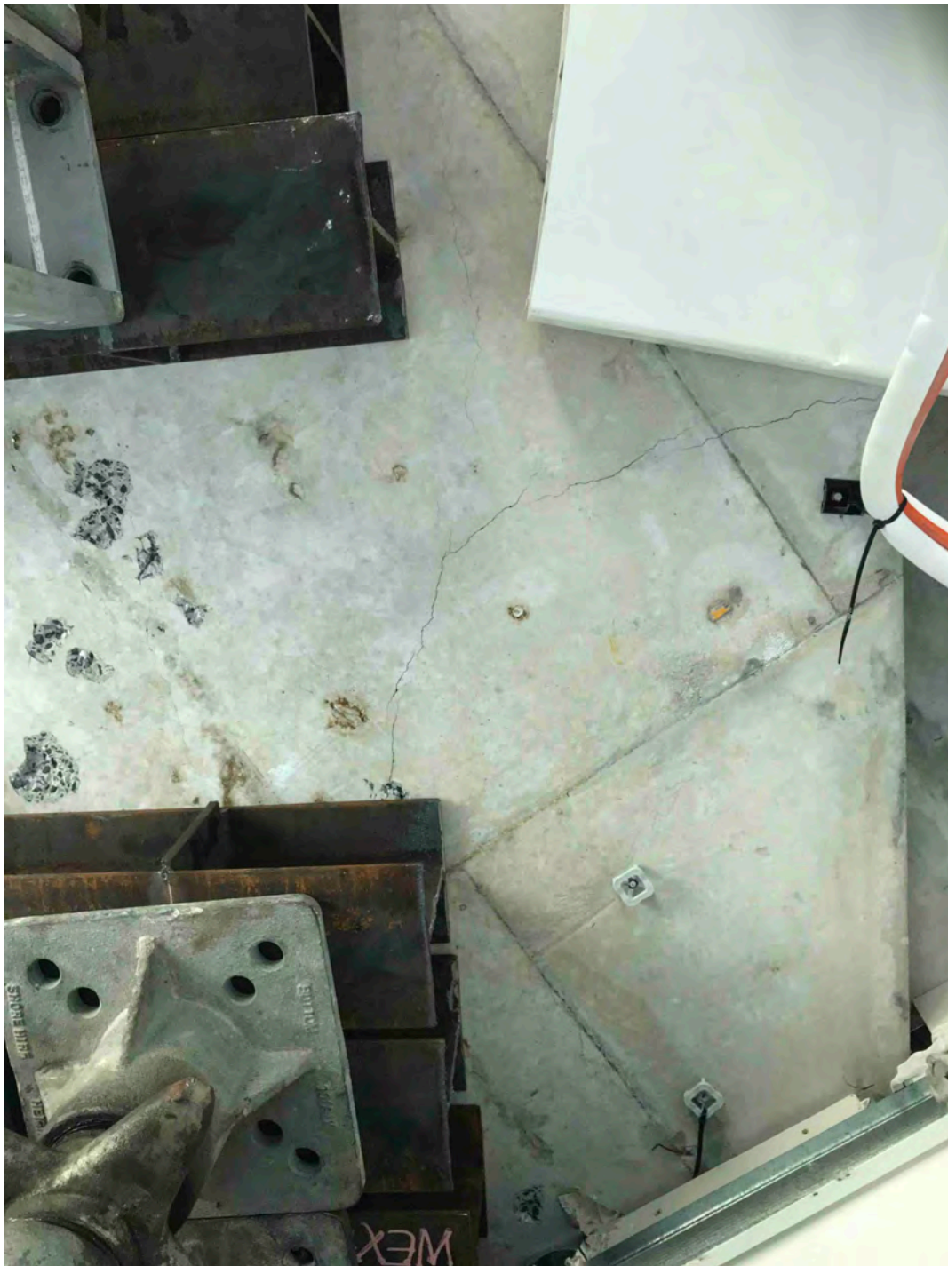
Figure 11. Photograph of a crack in the floor plate between Levels 3 and 4.
