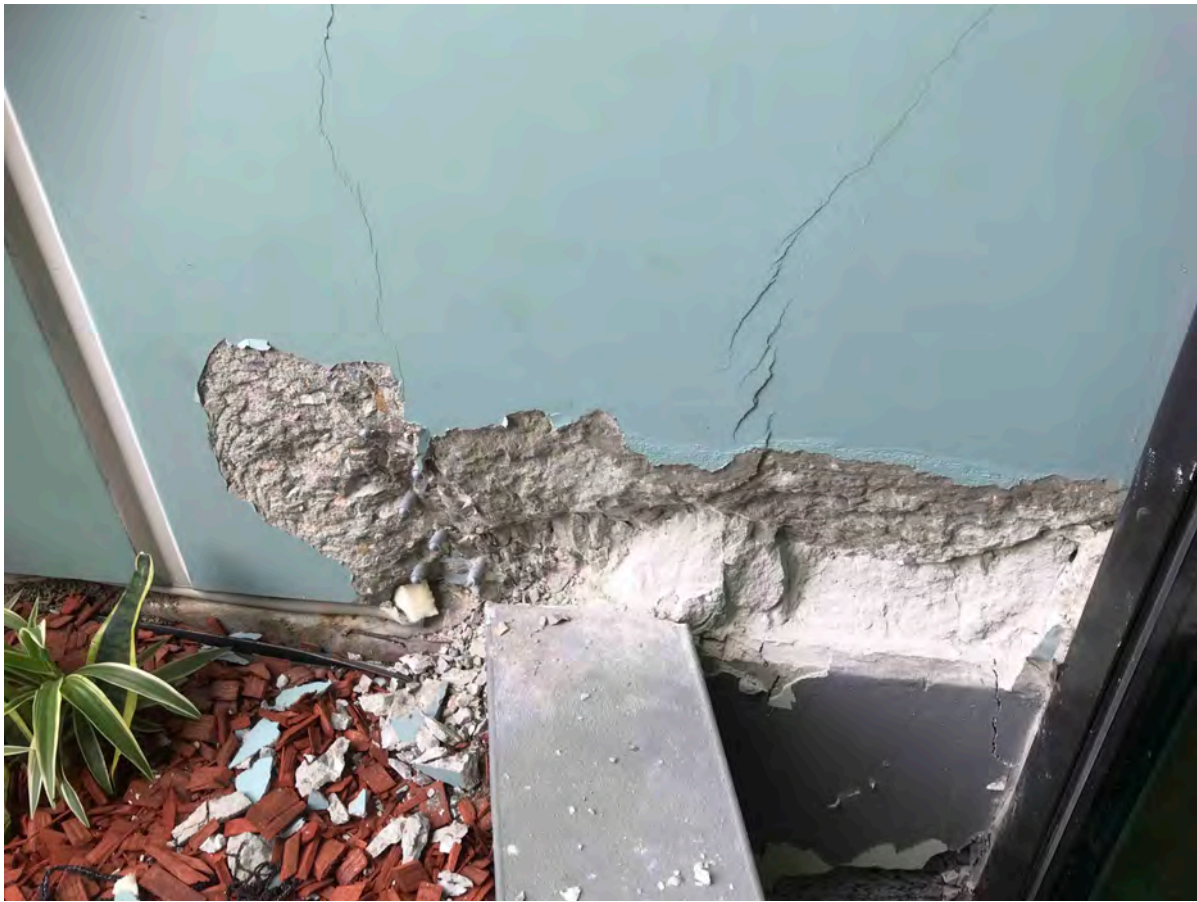
Figure 6. Damaged precast Panel A at Level 10 above column C38, after some broken sections of concrete removed.
