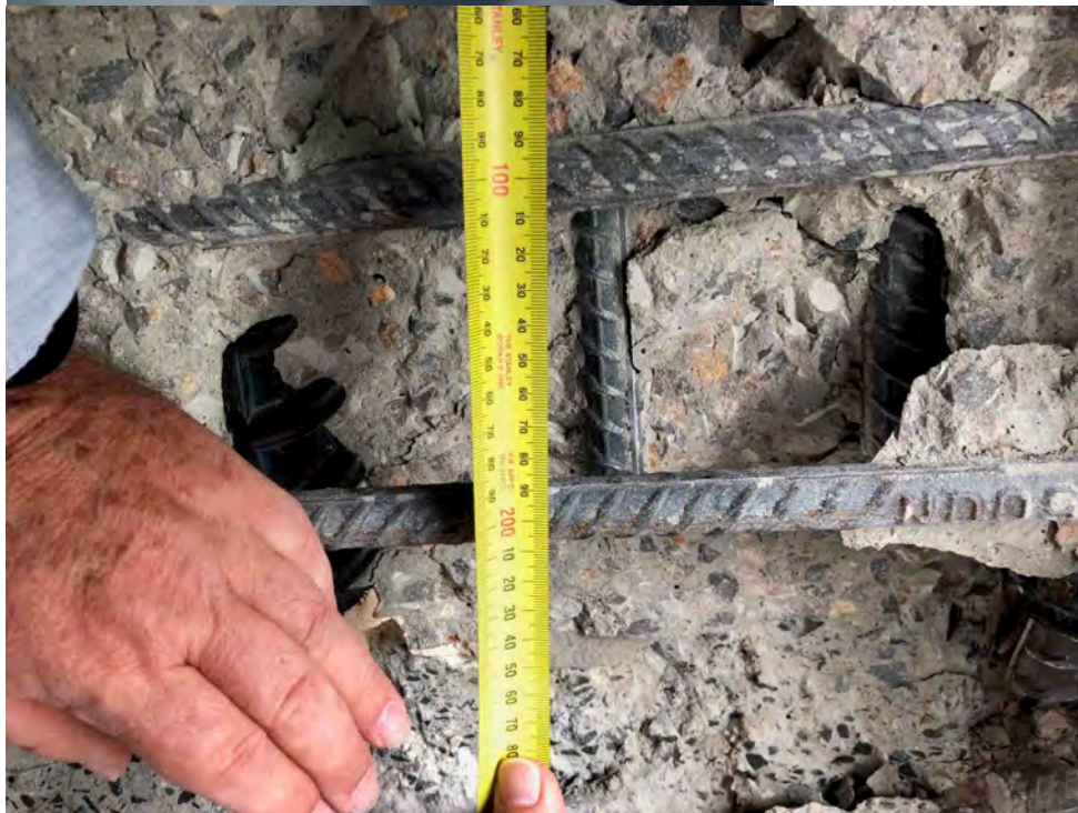
Figure 8. Photographs of the outside (top) and inside (bottom) of panel A at Level 10 just above hob beam adjacent to column 21, indicating N20 reinforcing bars at 100 mm centres in the lower portion of the precast panel. Note the exposed grout between panel A and the hob beam and the black plastic sheath for the joining dowel (top photo, right of tape measure).
