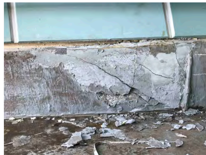
Figure 7. Photographs of the hob beam in the vicinity of column 38 at level 10, prior to pouring concrete (top photo), inside the building on 8 January 2019 after cracked concrete cover removed (middle), and outside on 8 January 2019 after the garden and waterproof covering removed (bottom). Note the positioning of the reinforcing bars, the encroachment of the column bars into the cover zone, the lack of anchorage of some horizontal bars, and the encroachment of a conduit into the concrete cover zone. The vertical dowel bars that engage with the precast concrete panels can also be seen in the top photograph.
