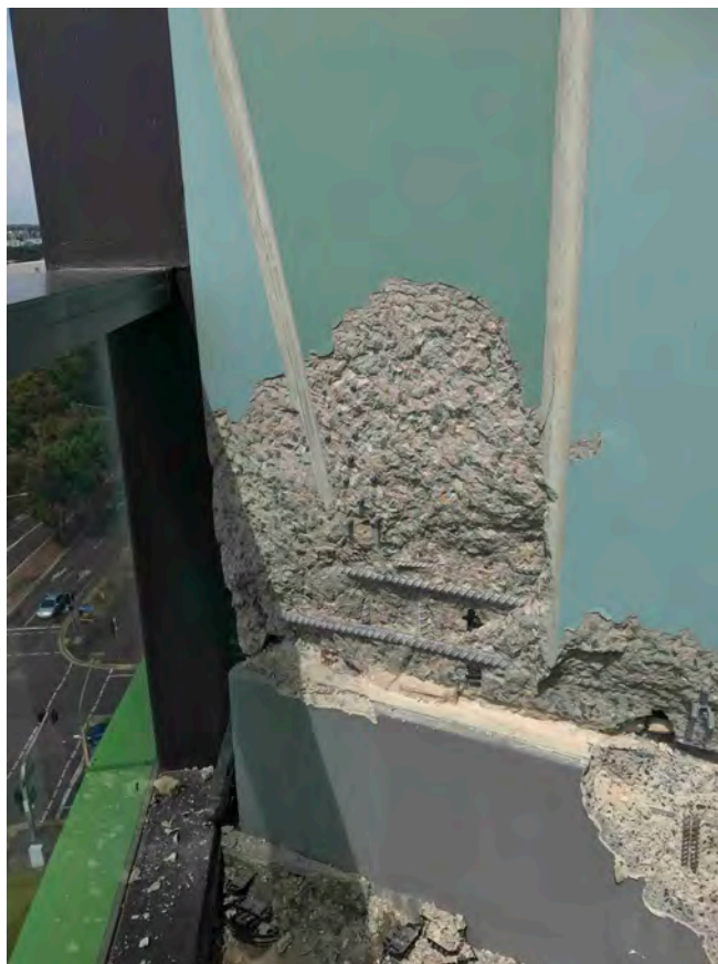
Figure 5. Damaged precast Panel A at Level 10 above column C21, before (top) and after (bottom) broken section of concrete removed.
