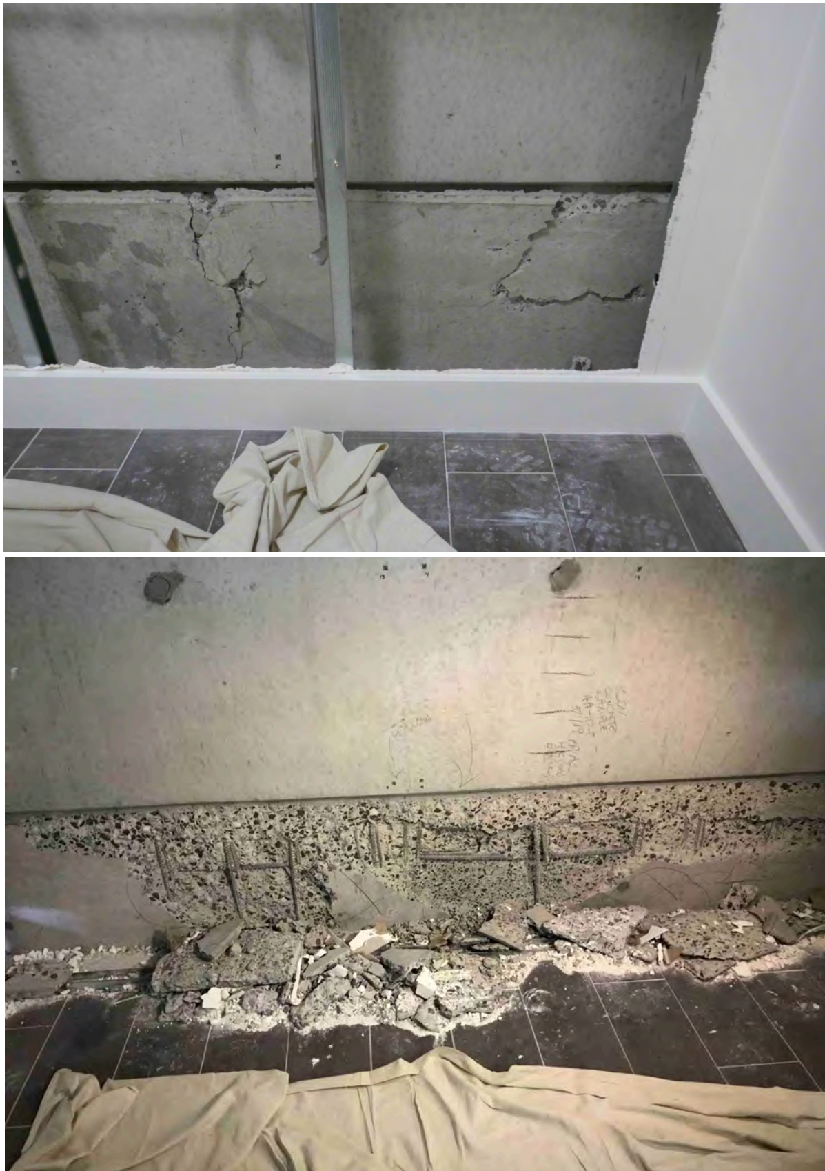
Figure 10. Photographs of the damaged hob beam on Level 4 near column C34 before (top) and after (bottom) cracked concrete removed.
